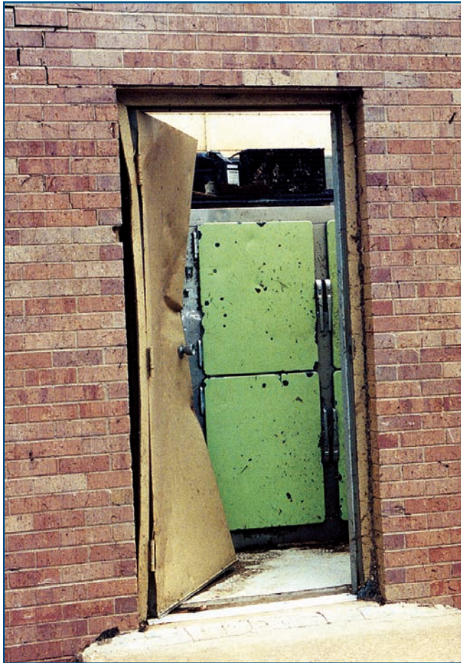
Figure 2-3 Example of severe damage from a windborne missile. This metal door was pushed inward by the impact of a heavy object.
